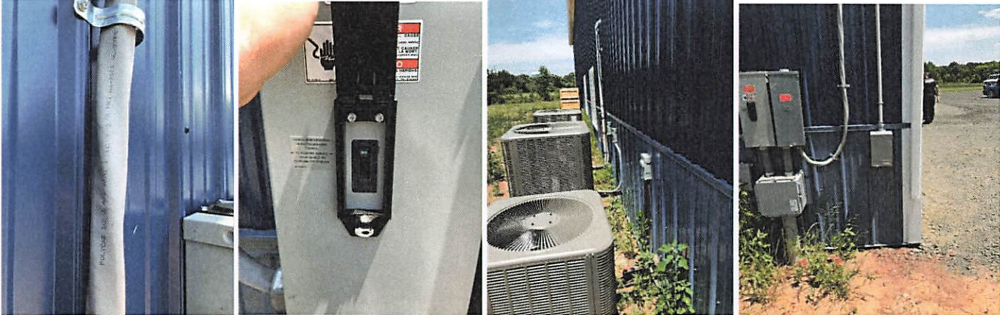
4/0AL cable, probably sized adequately but is only rated for 180 amps. Residential structures allow for exception with out load calculations.
