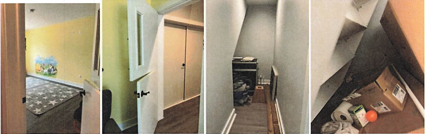
NM cable installed without physical protection, under. Stair protection not installed.
