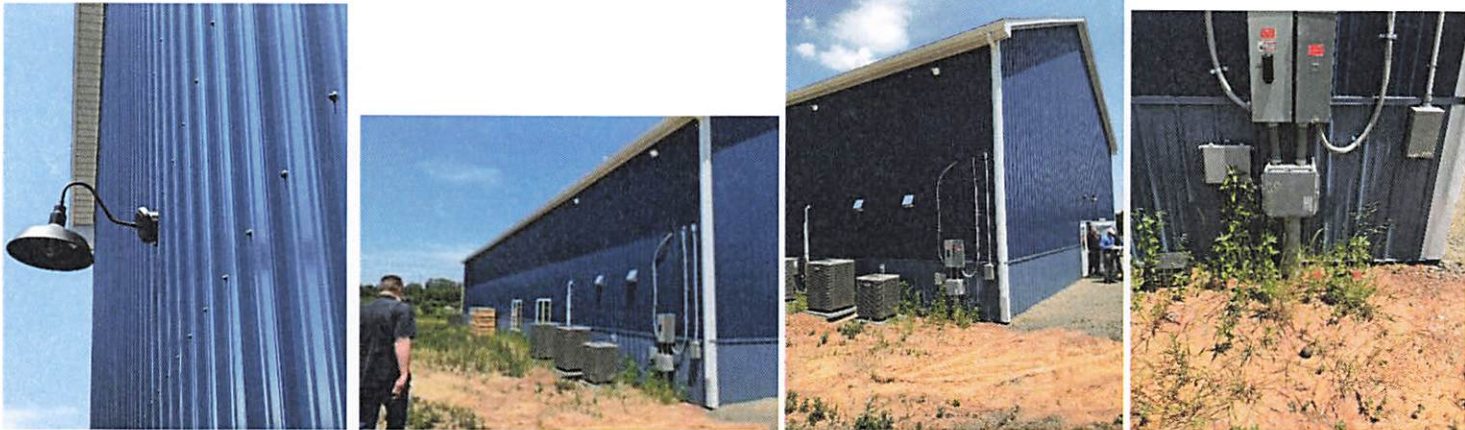
Exterior light not installed properly.
