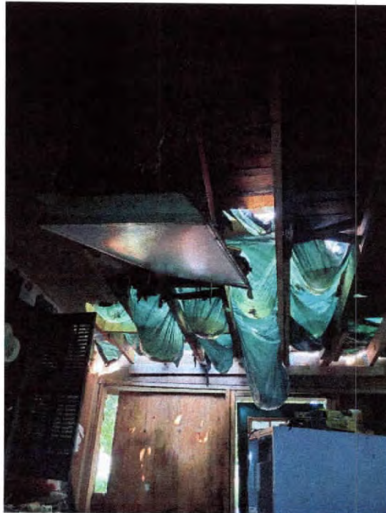
Figure 4 – Kitchen Ceiling/ Wall damage
