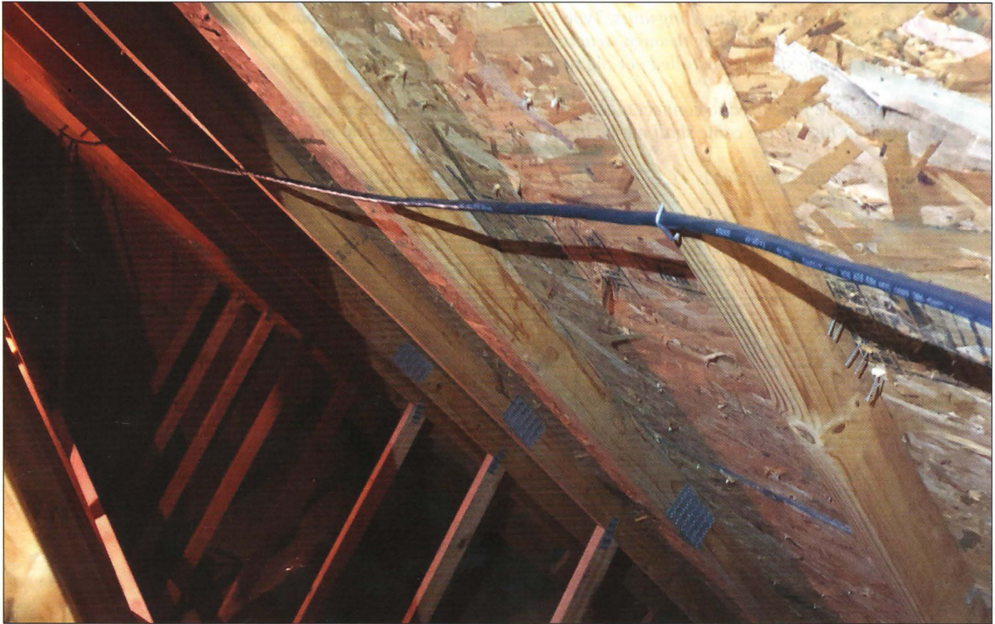
Photo 3. Interior TC-ER cable installed under the 2017/2020 NEC should be secured every 1.4 m (4 ½ ft). If a firefighter saws through the roof with a chainsaw (a thing they do), that there is a chance they hit the cable that is stapled to the rafter. To prevent this mishap, the firemen should disconnect the service prior to venting. PV conductors in buildings have to be under 30 volts within 30 seconds of being disconnected [690.31(B)(1)]. For systems connected on the load-side (i.e. through the circuit breaker), turning off the main breaker also disconnects the PV circuits. For systems connected to the line-side, the firefighter will separately disconnect the main service and the PV service. Pulling the meter shuts down all the services in either case.
