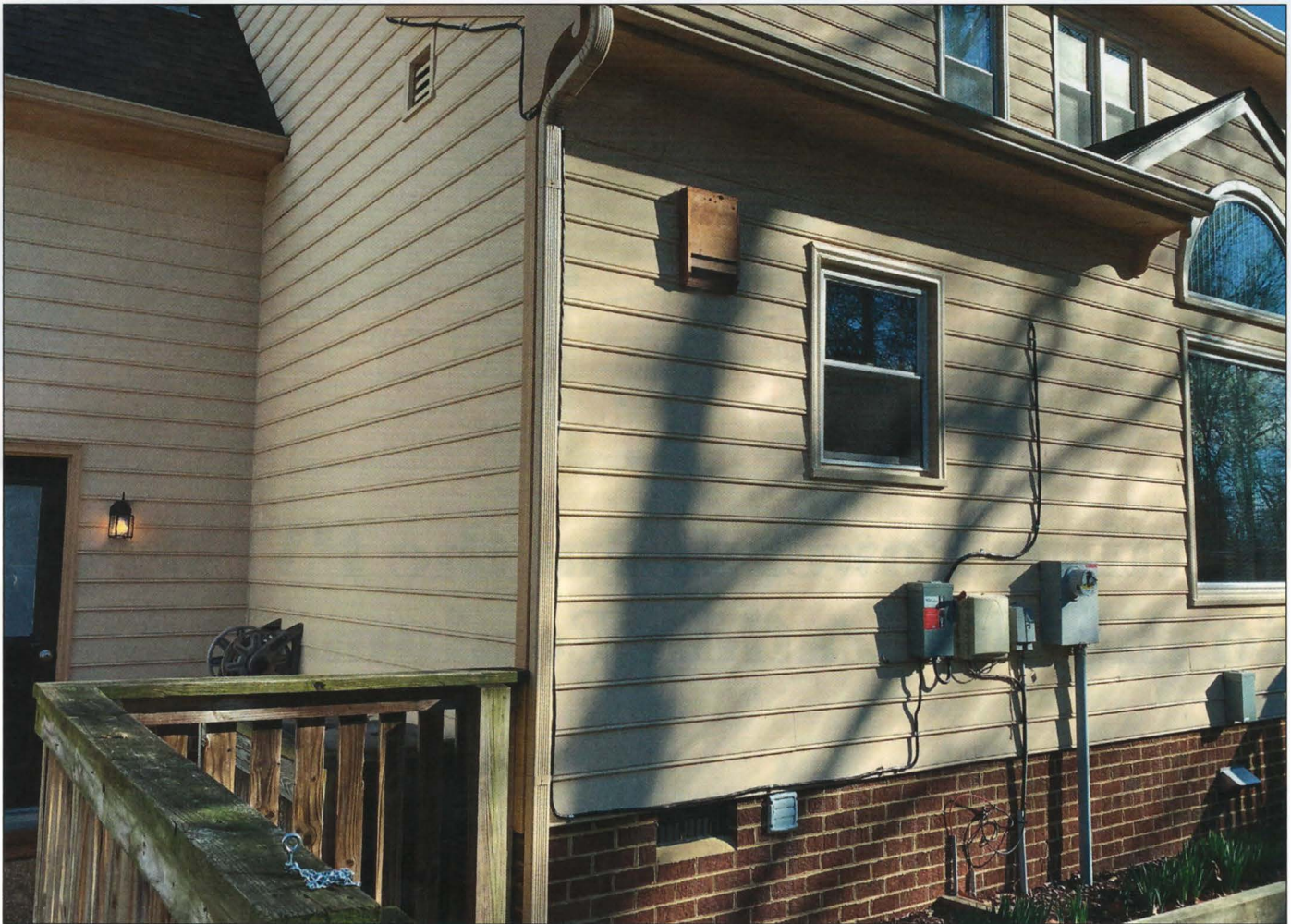
Photo 4. Exterior runs of TC-ER cable on a single-family dwelling
