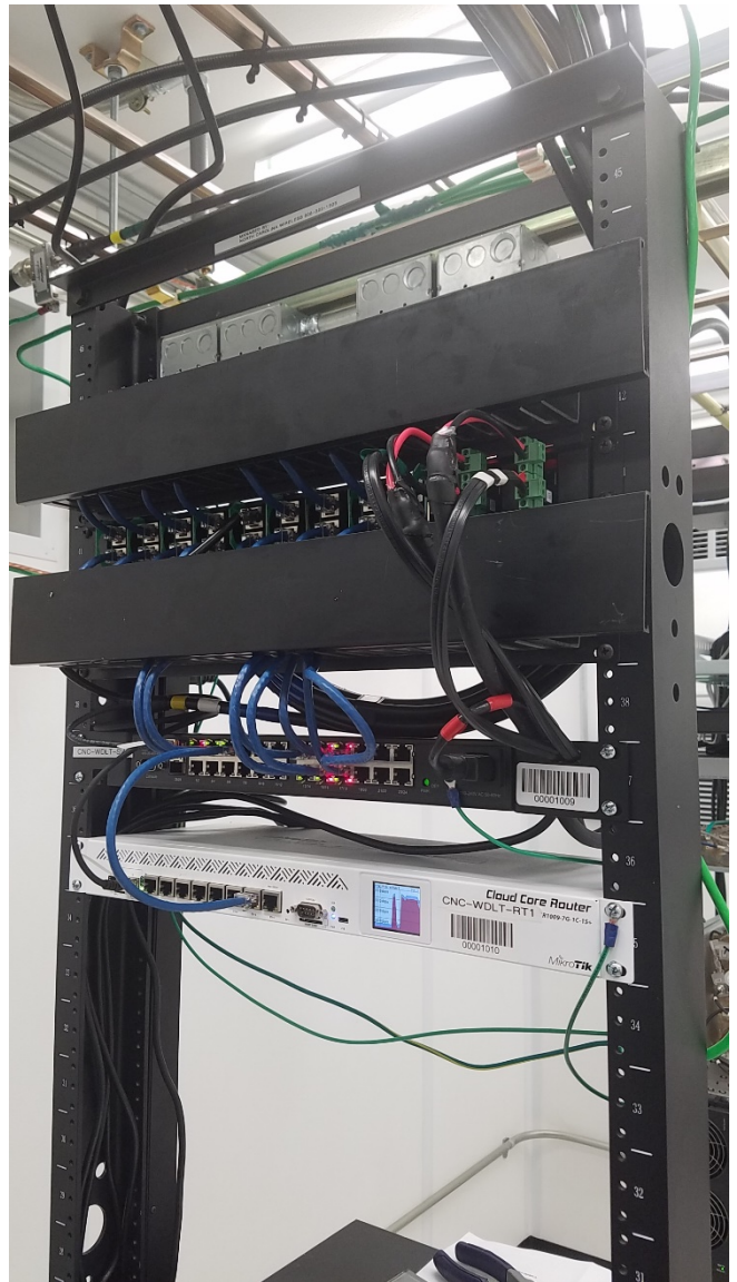
B. 2-Post Tower Rack in Person Co NC
