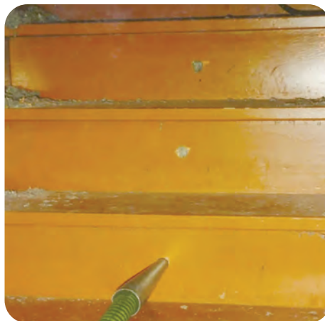
11. If backside of stairs is sealed, blow insulation into cavity behind stairs
