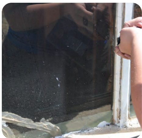
1. Remove all broken glass
